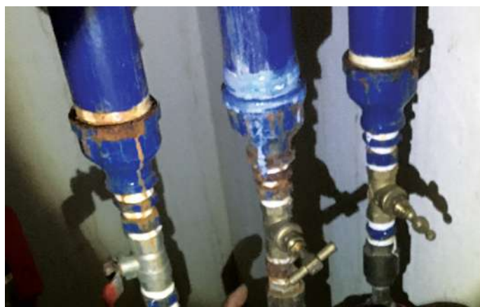
Figure 5: Corrosion on metallic pipes
