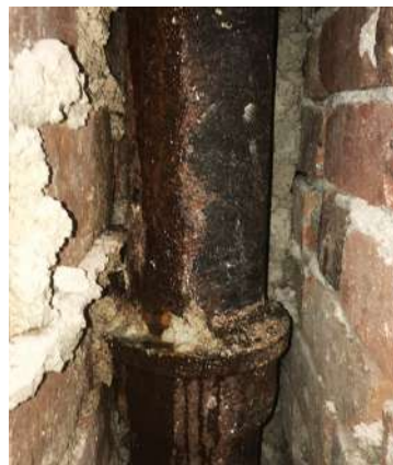
Figure 13: Leaking rusty cast iron pipe
