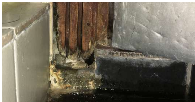
Figure 2: Rotting of timber door frame at bathroom
