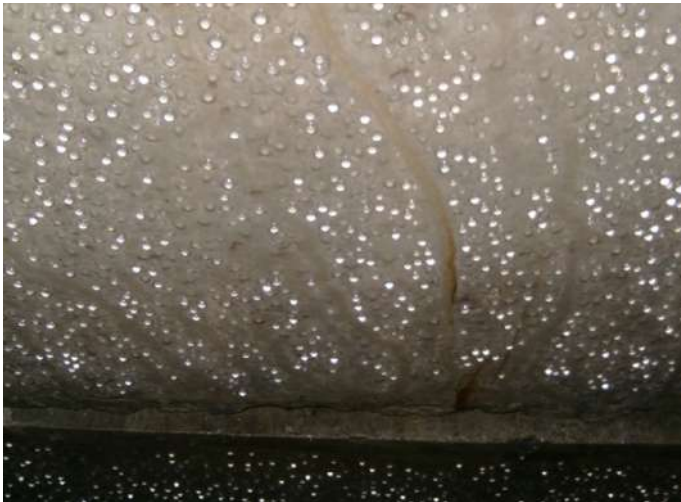
Figure 24: Condensation on RC slab
