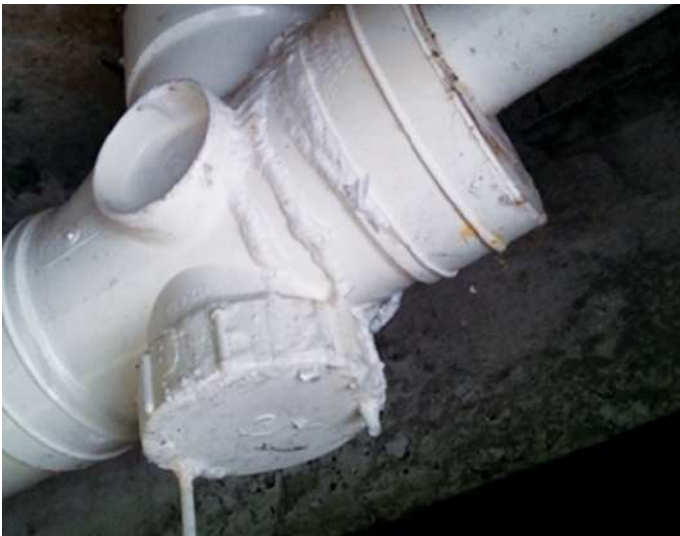
Figure 15: Efflorescence due to waterproofing failure
