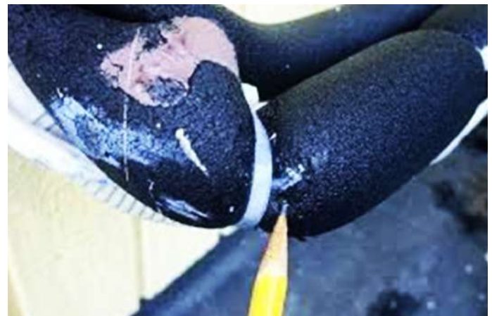
Figure 25: Poorly insulated copper pipes
