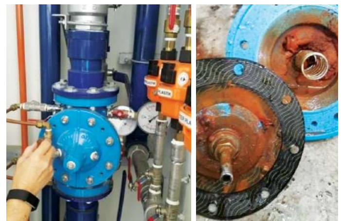
Figure 6: Pressure reducing valve (PRV)
