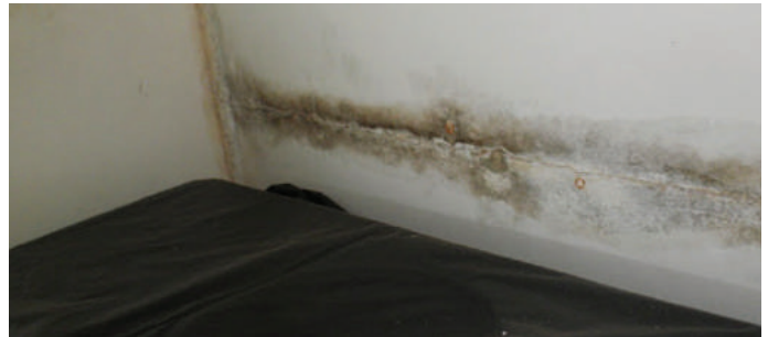
Figure 1: Wall exposed to dampness
