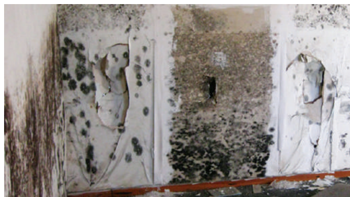
Figure 3: Hazardous microbial growth in indoor spaces
