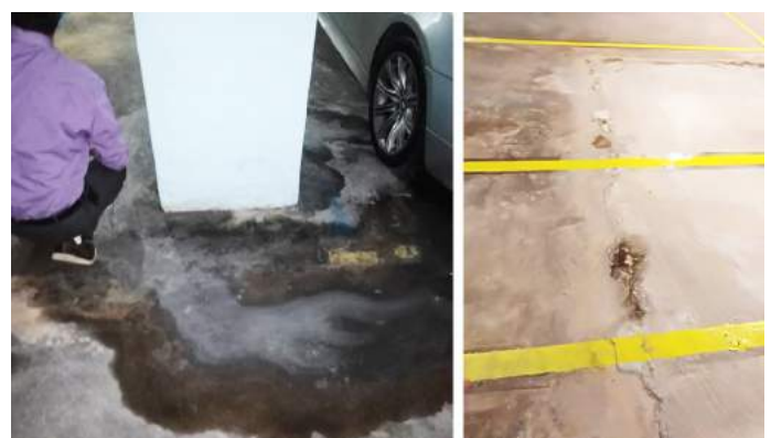
Figure 5: Water seepage in basement floor due to rising water table
