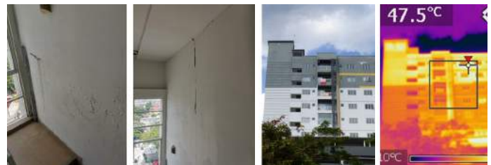
Figure 4: Heat induced cracking on walls and facades at the highest floor with flat roof
