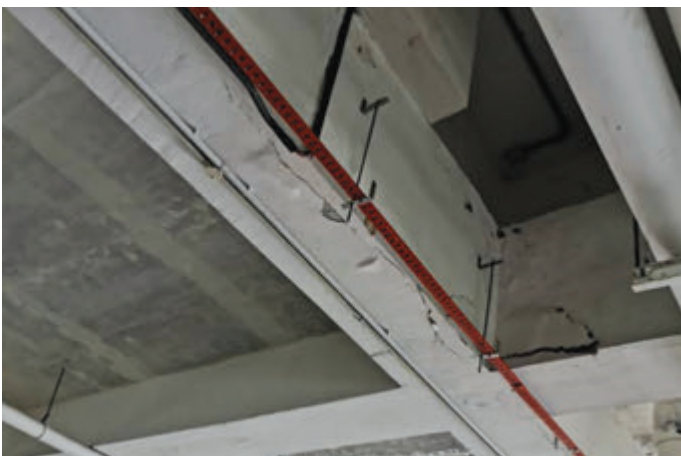
Figure 1: Latent Defects under swimming pool in a 4 year old condominium
